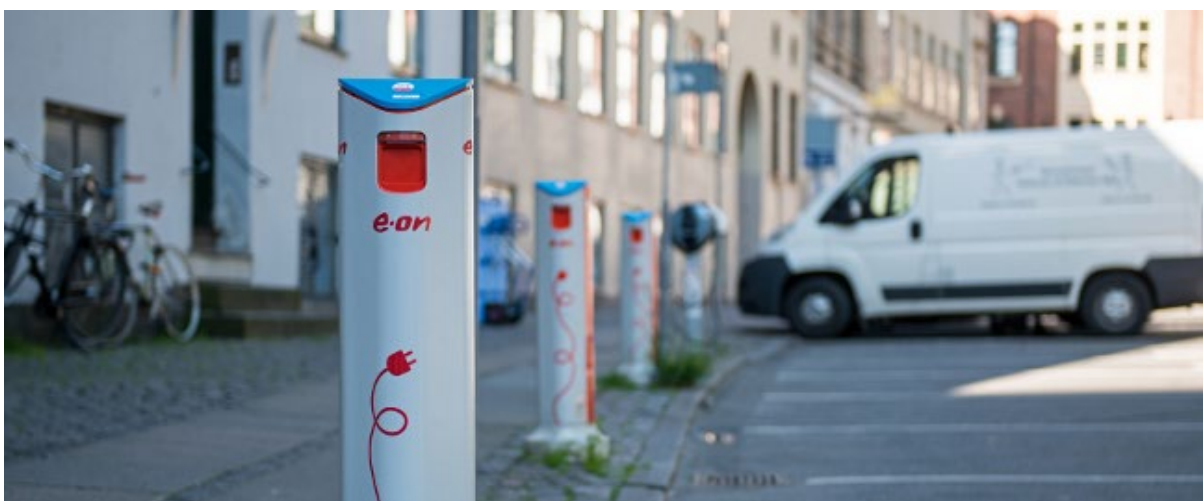
E.ON EV-Charger in Sonderborg. Credits@Sonderborg
